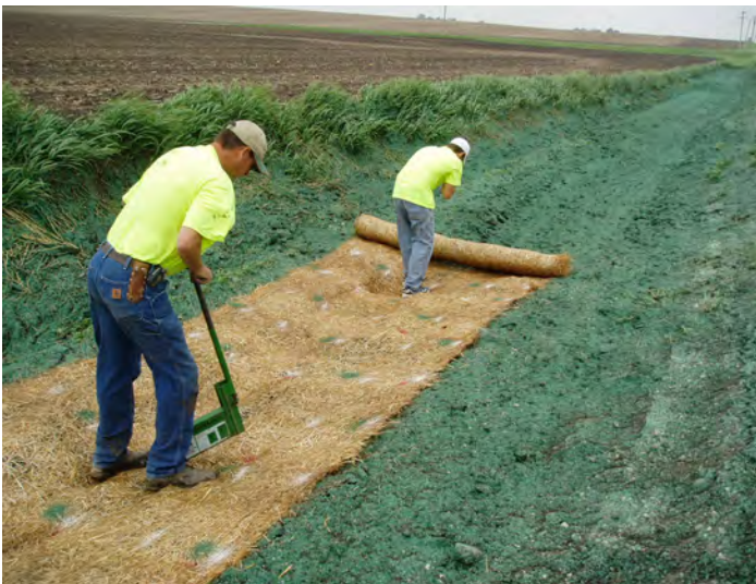
Roadside technicians install erosion mats in Dallas County. Photo courtesy of Kirk Henderson.
